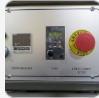
Variable Air Velocity Control
